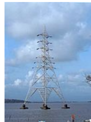
This electrical pylon is a three-dimensional truss structure
