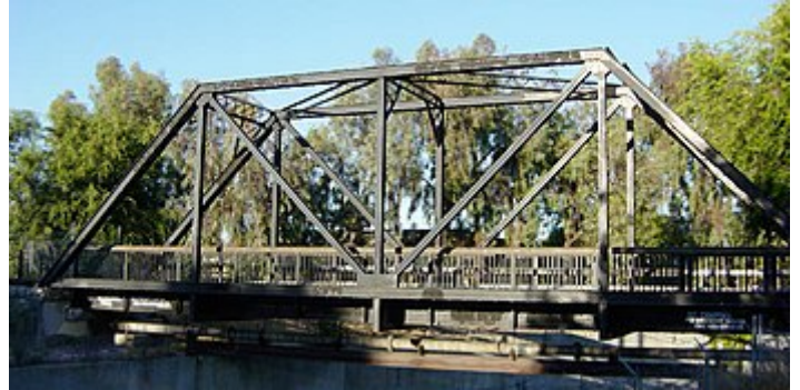
Truss bridge for a single-track railway, converted to pedestrian use and pipeline support. In this example the truss is a group of triangular units supporting the bridge.
