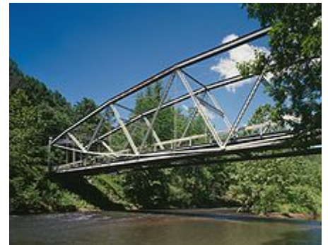
The Waterville Bridge in Swatara State Park in Pennsylvania is a lenticular truss
