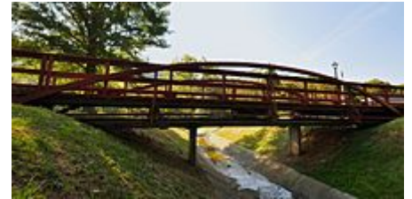
A bowstring truss is used on the oldest metal bridge in Virginia
