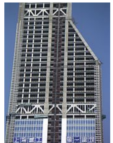
Truss sections stabilize this building under construction in Shanghai and will house mechanical floors
